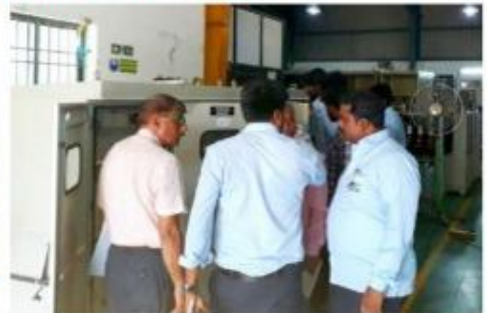
Successful inspection of VCB panels by Megha Engineering & Infrastructures Limited
