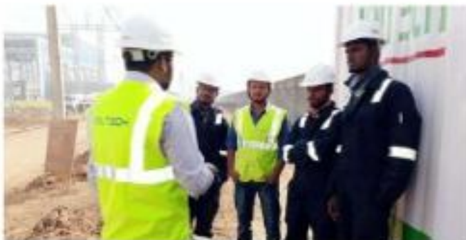
ABB- HVDC- Raigarh, ICD1 (HVDC)
