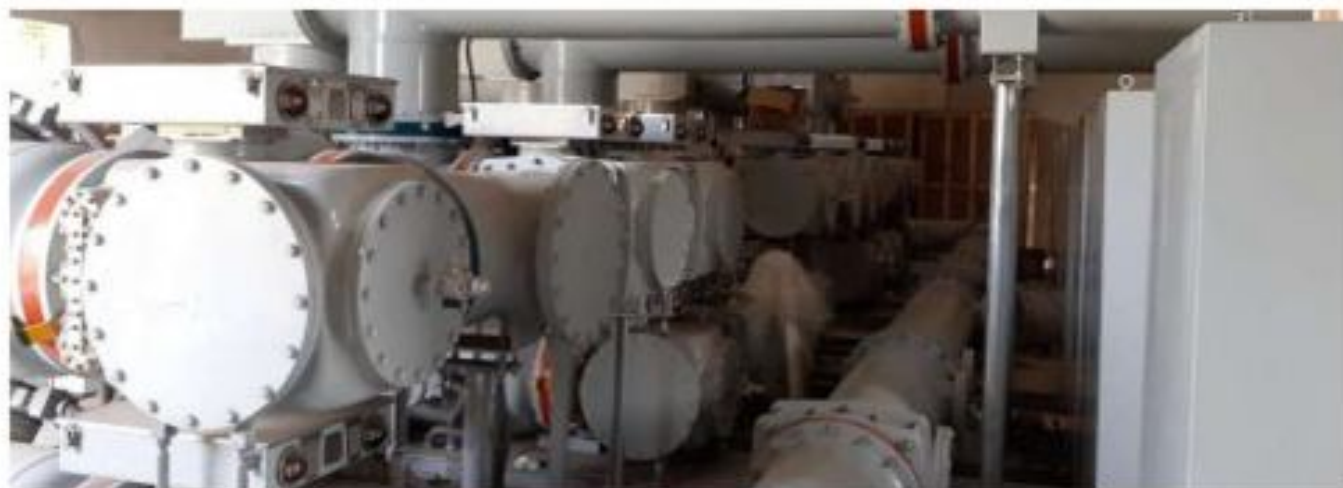
132/33kV GIS at Orlu, Nigeria.
