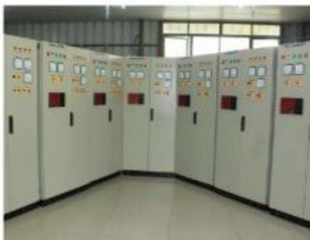
Successfully inspected and supplied 12 nos. of 110V Battery Chargers
